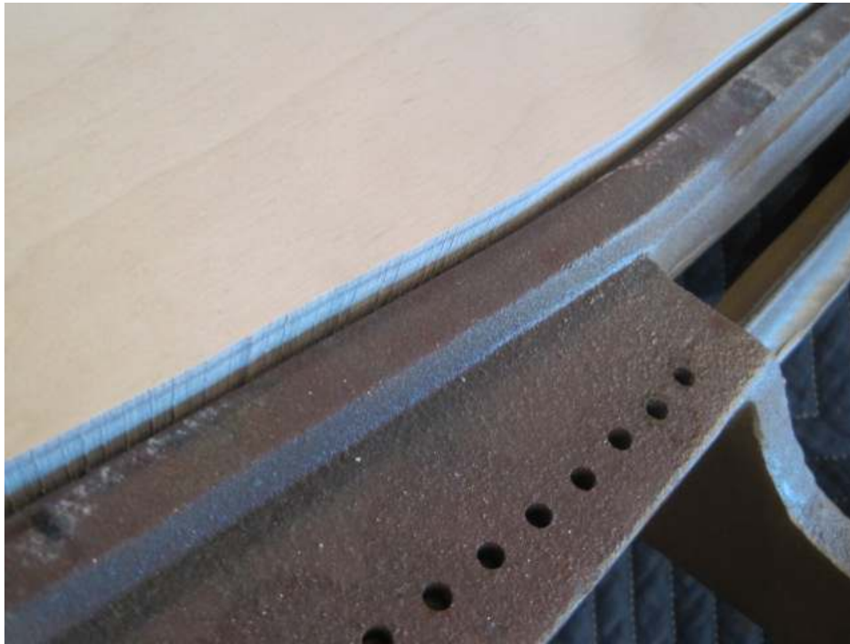
Photo 55: Out of the gate, there are plenty of gaps. With the irregular contour of the cast iron flange, this is about par for the course when using a band saw to make the cut. The factory can do better on the first pass, taking advantage of computer operated, highly specialize cutting equipment.
