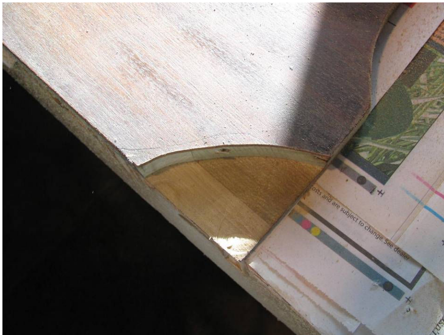
Photo 3: A much more fixable repair
